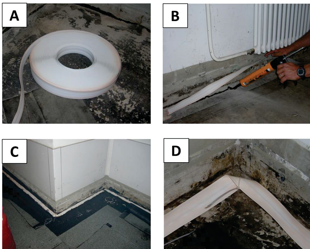
Figure 3.13: A shows the flat ribbon cable on a spool. The cable is cheap and easy to handle. B shows how the cable is glued to the concrete floor to avoid that water can flow under the cable without direct contact to the cable surface. C shows how the cable is installed along the outer walls of the building and D shows how the cable is bent around corners. Bending the cable also distorts the measurement signal and causes partial reflections. Therefore there should be only one corner per cable to ensure that the signal still can be evaluated.
