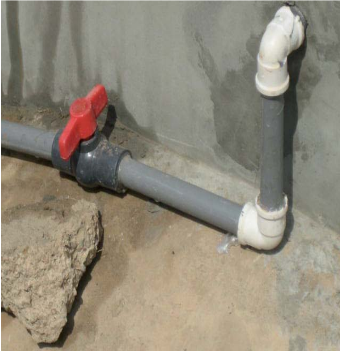
Fig.6: The Piping of the gas
