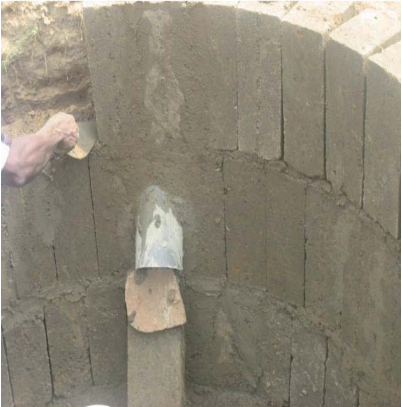
Fig. 2: The Construction of the digester walls and the fixing of the pipes.
