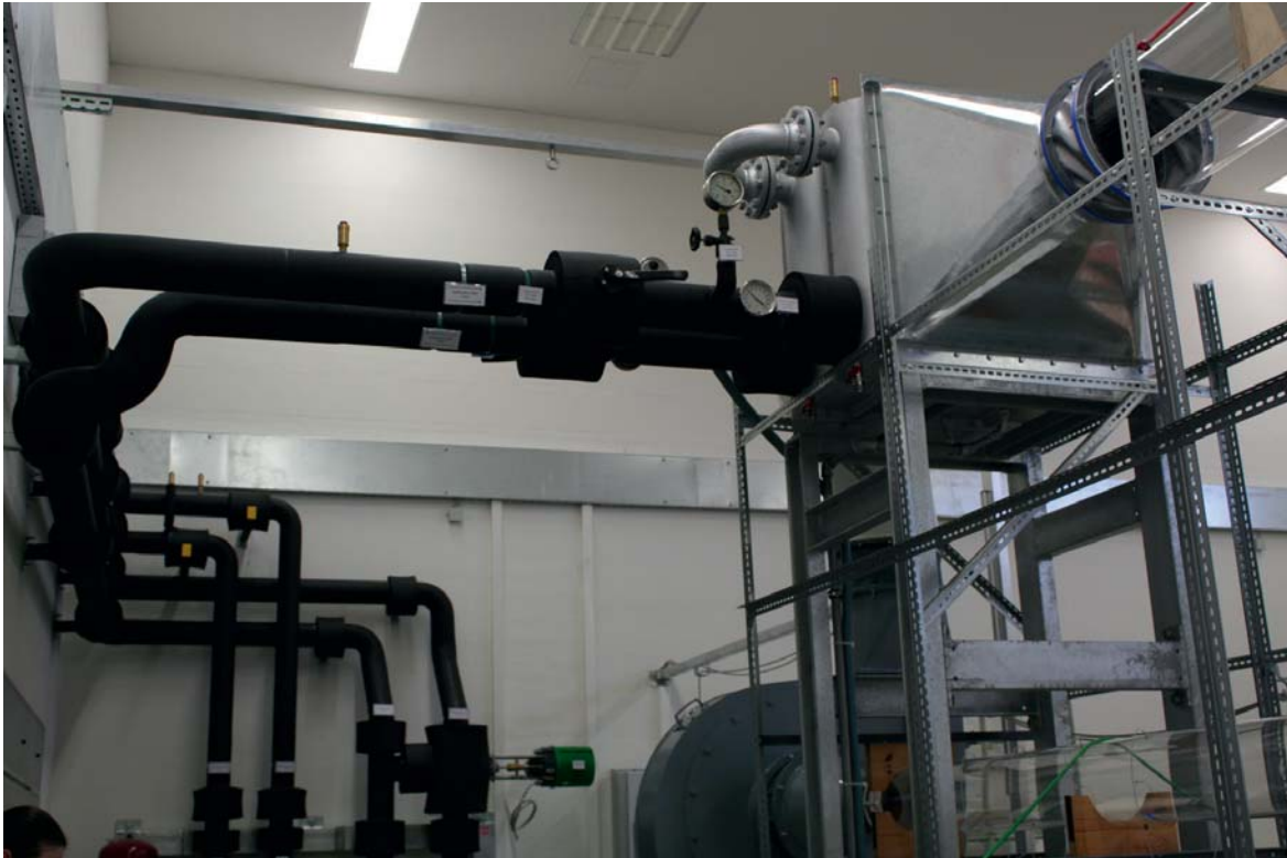
Figure 4.8: Cooling system with heat exchanger (top), piping system (black pipes), pressure control system, valves and accessories.
