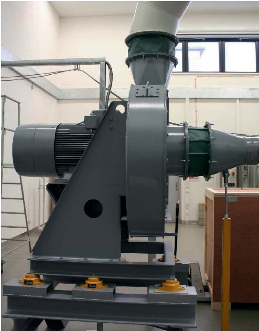
Figure 4.9: Centrifugal blower with motor and blower support equipped with damping elements. Coupling parts between blower and suction side, and blower and return line to avoid transmission of vibrations.
