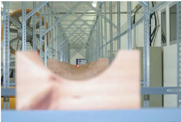
(a) Sub-construction of the CoLaPipe with a laser point at the end marking the position of the blower unit. The theodolite and the surveying level are used to set up the sub-construction as well as to establish the connection to the blower unit.
