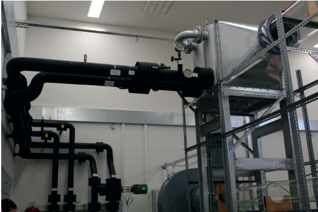
Figure 4.12: Cooling unit with accessories and piping system.
