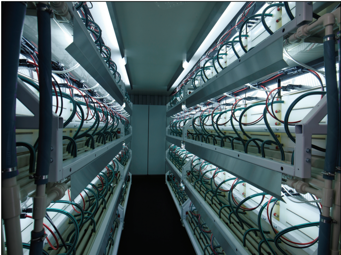
Figure 1-7: Interior view of a Gildemeister CellCube container; Copyright by Gildemeister Energy Storage GmbH, used with permission
