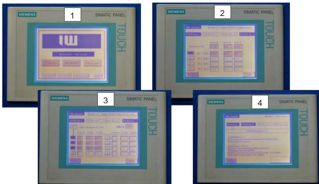
Fig. 36: Primary PLC control system
