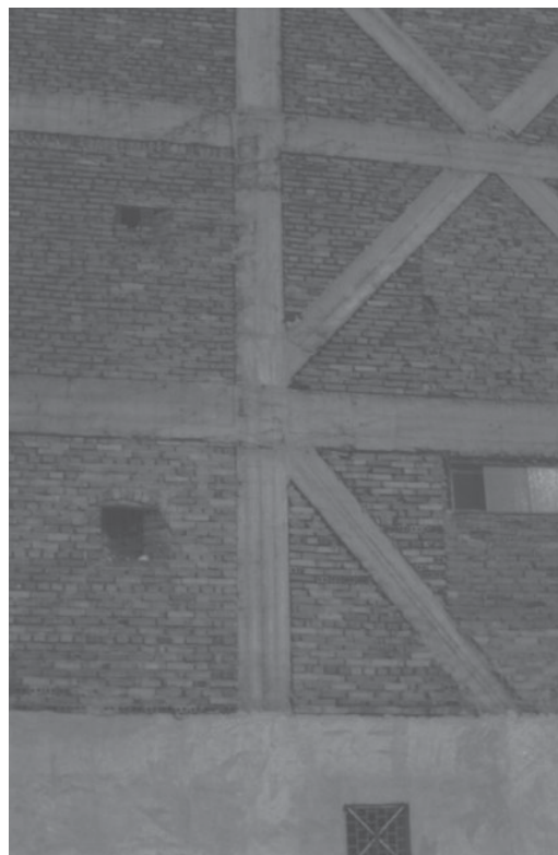
Figure 4.8: Detail view of reinforced concrete diagonal braces within a reinforced concrete frame structure for a building in Bucharest
