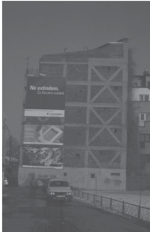
Figure 4.7: View of a building in Bucharest with reinforced concrete frame structure and diagonal braces
