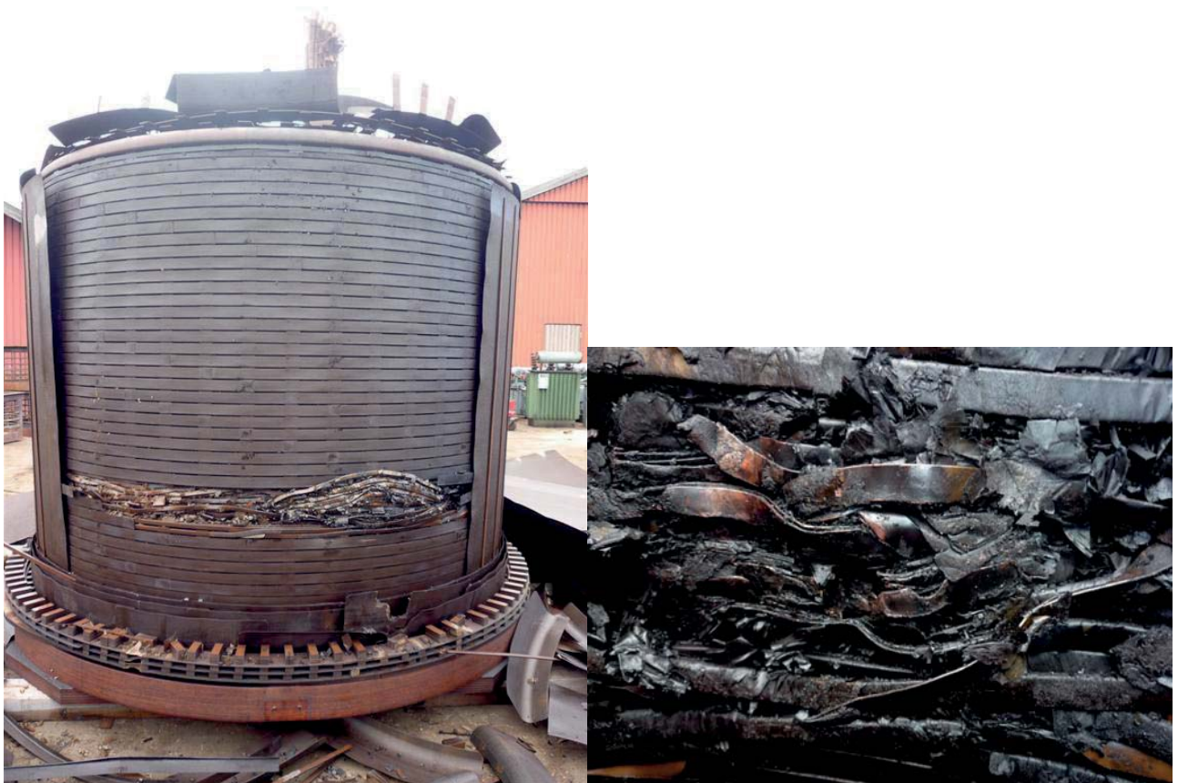
Figure 1.1: Effects of flashover due to a dielectric fault in a transformer coil
